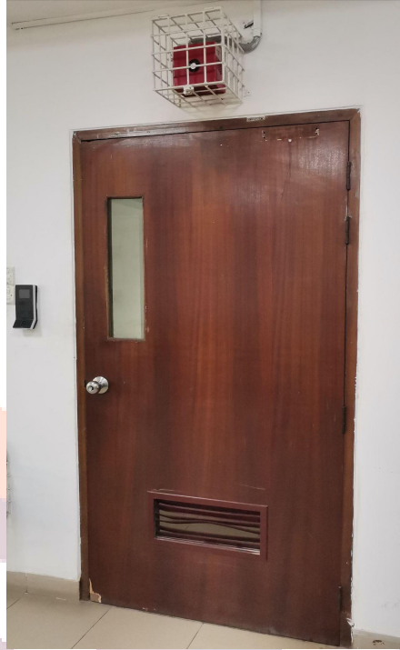
Figure 6. Classroom entrance door featuring a built-in loupered ventilation grille, with a sensor node installed just above it for capturing air exchange data.
